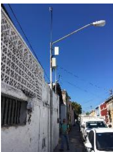
Over 70 units of A2 & A2-Ei are mounted on lampposts to provide outdoor WiFi
