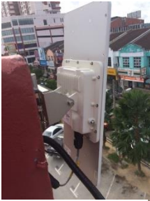
A2-Ei's are mounted in the outdoor areas to provide large coverage
