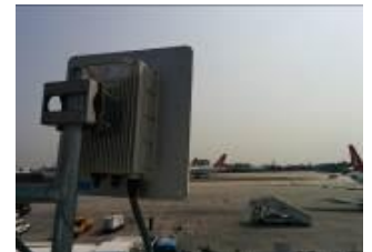
Installed Altai A8-Ein on lamppost in the apron areas
