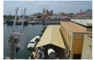
Altai A2 and A3-Ei were installed on the rooftop to provide outdoor coverage
