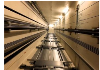
Elevator shaft is a challenging environment for wireless network
