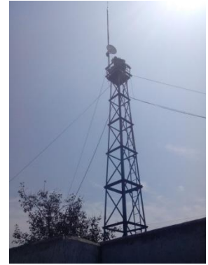
C1n & C1an are mounted on towers to provide WiFi coverage
